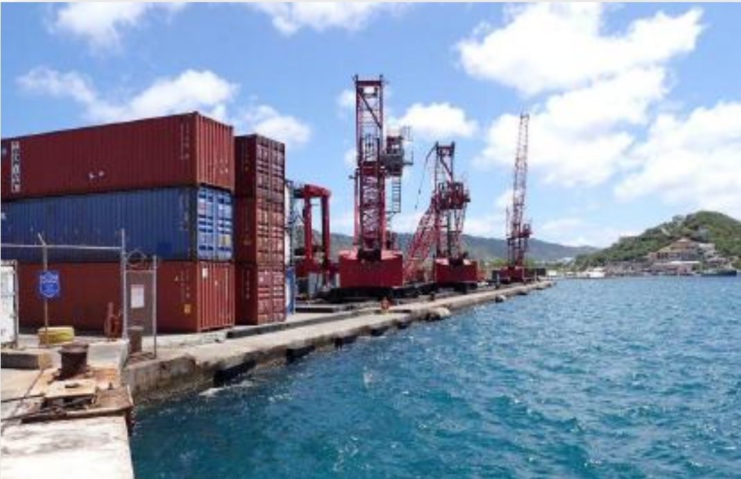
Crown Bay cargo dock deterioration
