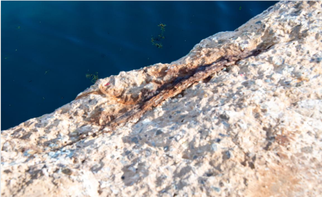
Crown Bay cargo dock deterioration
