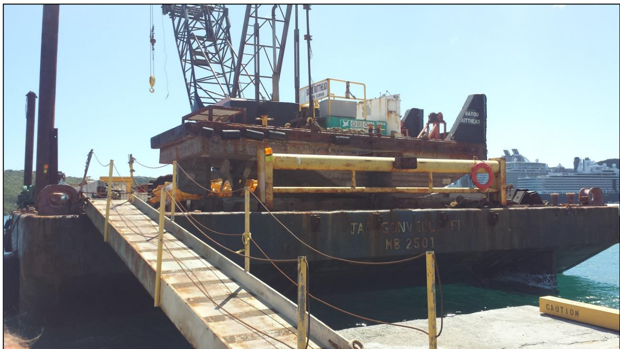
The barge operated by Orion Marine Construction, Inc. is stationed in Crown Bay as workers prepare the silt curtain to begin dredging.
