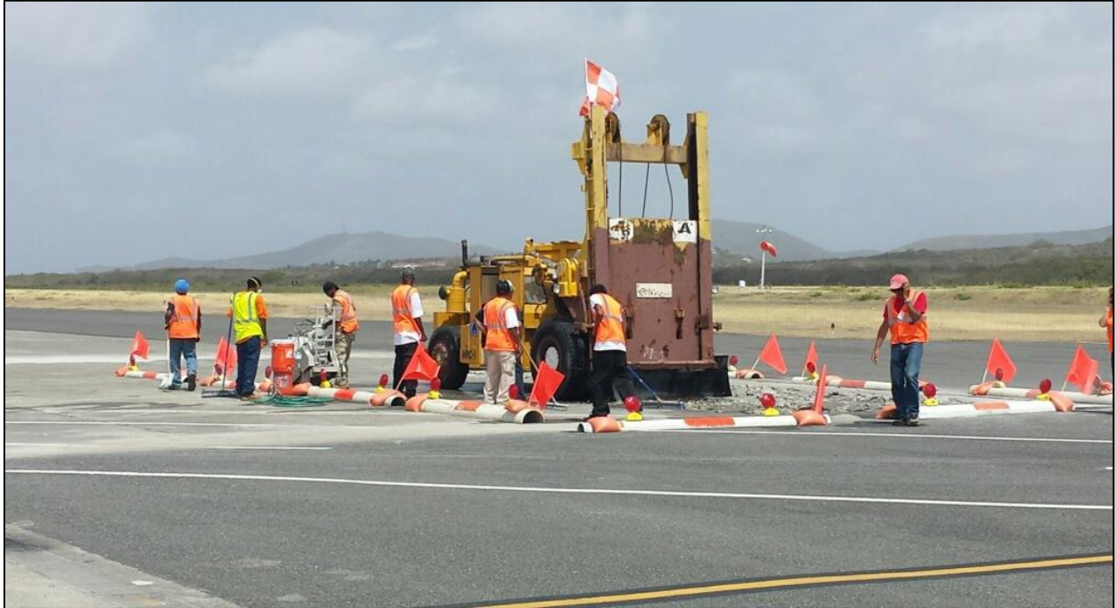
Betterroads Asphalt Corporation, LLC. was hired by VIPA to complete Phase 2 of the HERA Apron Rehabilitation Project on St. Croix.
