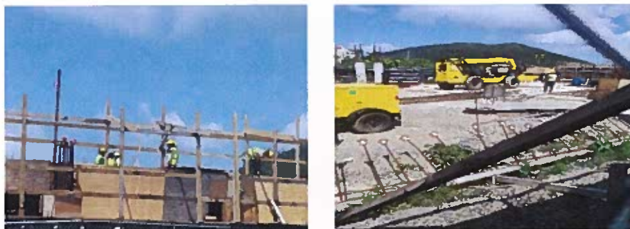
Work has resumed on the two-story parking garage at Red Hook, St. Thomas. Expected completion – July 2018.
