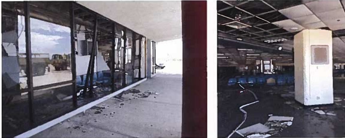
Cyril E. King Airport Terminal Post Hurricane Irma
