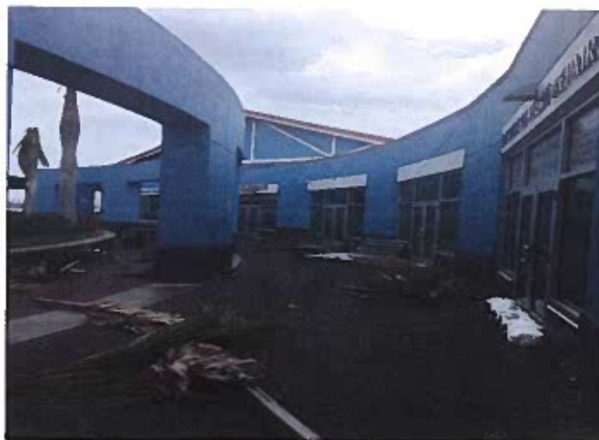
Damaged Crown Bay Center Storefront
