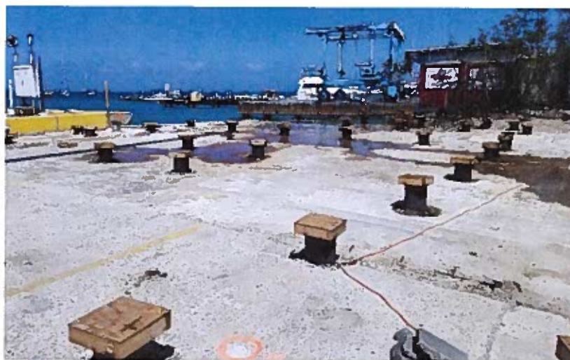
The pile casings for the new Passenger Terminal have been installed. Expected completion – December 2018
