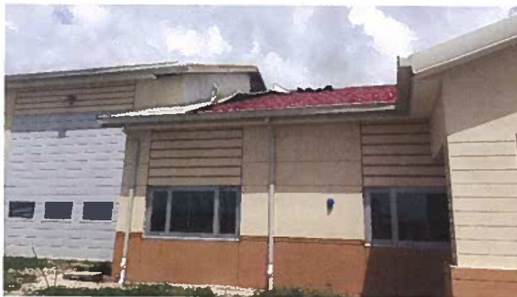
Damaged Roof of the New HERA ARFF Building will be repaired by April.
