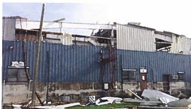
VIPA's Cargo and Office Building at the Container Port damaged by Hurricane Maria
